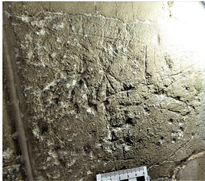
Fig 5. South doorway east side. Degraded baptismal crosses and other degraded marks. Photo KW38
